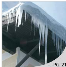
Roof & Gutter De-Icing
